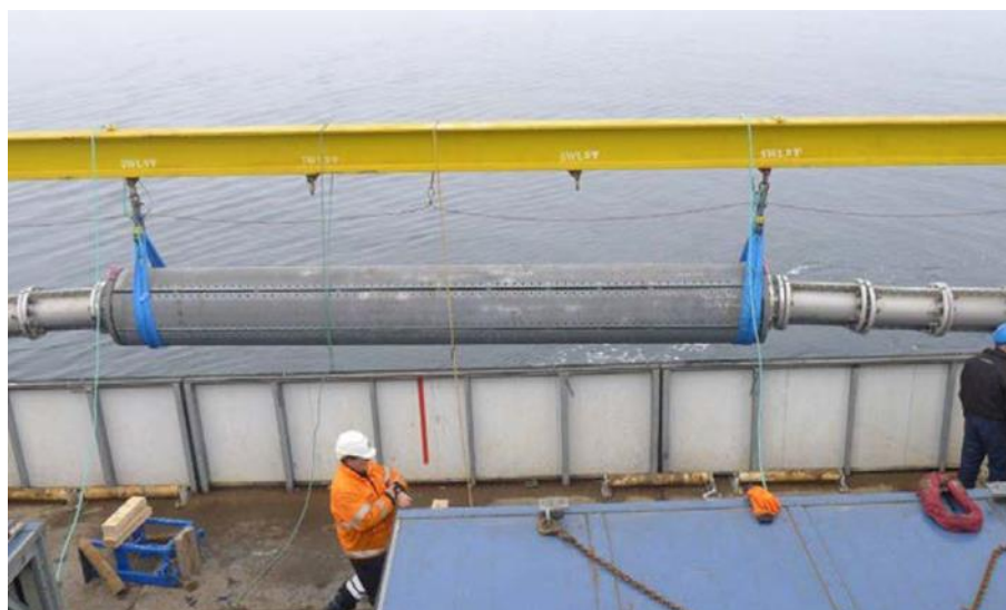
Figure 11 Rigid joint in a submarine cable and the support structure used for laying the cable [23]
